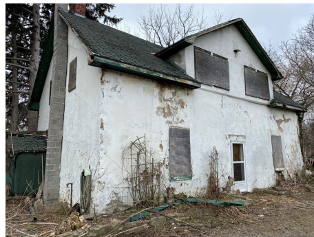
Damaged wall and missing gutter
