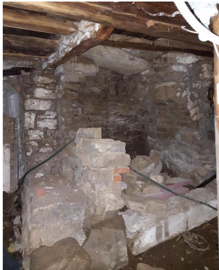
Figure 14: Chimney base on the north foundation wall with remnants of a relieving arch at far right (2017).
