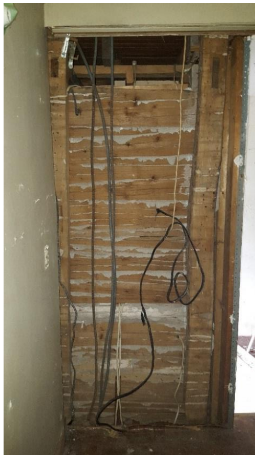
Figure 10: Partition of split-board lath-and-plaster between two hewn studs near the south entrance (2017).
