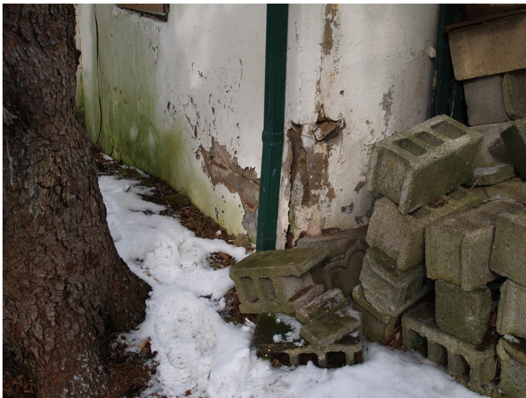
Figure 22: Mature tree growth near the southwest corner. Note spalling on the wall (2018).
