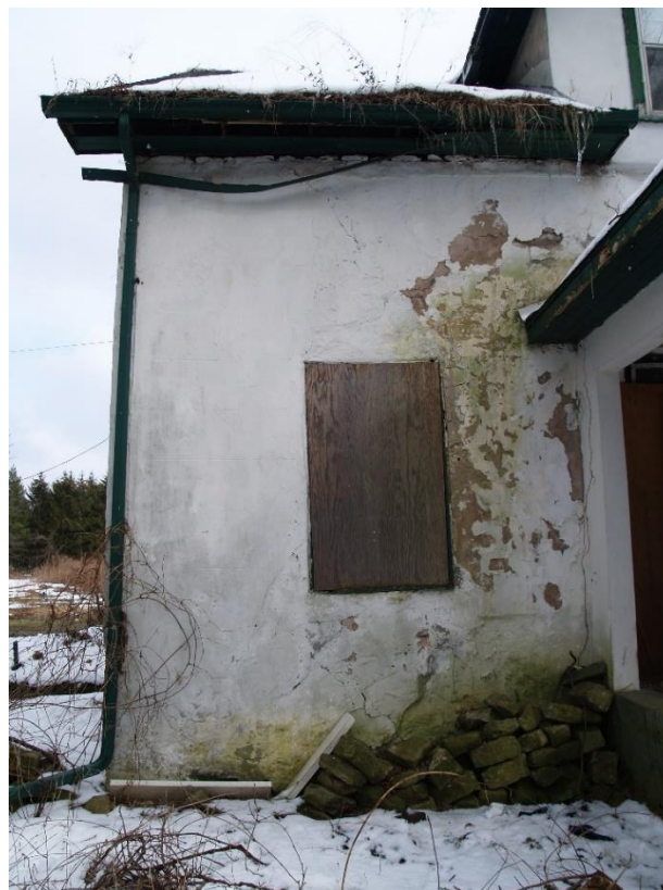
Figure 18: Evidence of wall movement at the northwest corner, just below the window opening (2018).
