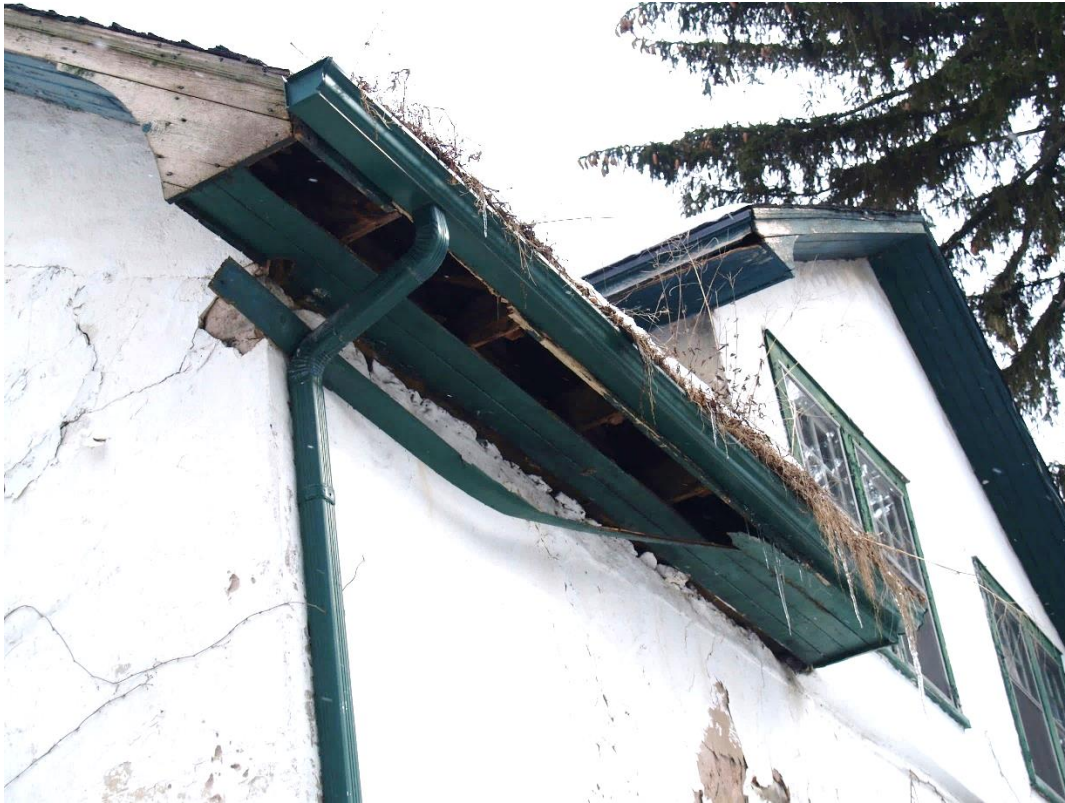
Figure 19: Vegetation growth in the gutter and lost and deteriorated fabric at the soffit (2018).
