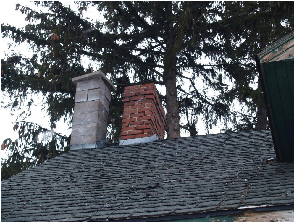
Figure 23: Chimneys in poor condition with inadequate flashing (2018).
