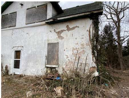
Damaged exterior wall
