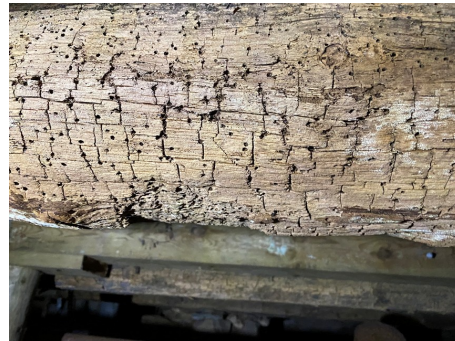
Damaged floor joists
