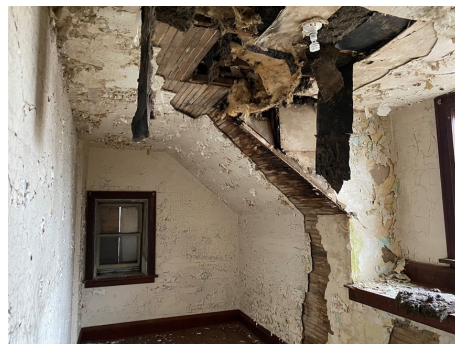
Ceiling damaged due to roof leak
