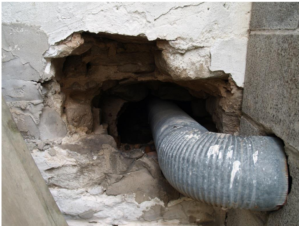
Figure 20: Poorly executed breach in the south end wall (2018).
