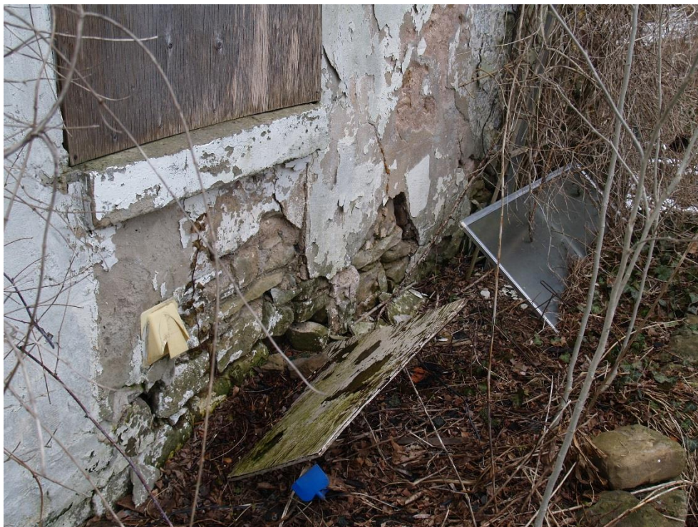
Figure 21: Render failure, mortar washout, and Portland cement repair (far left) under the north window on the east façade (2018).
