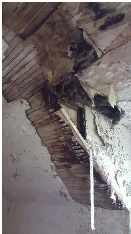
Figure 24: Water infiltration and damage to the lath and plaster surrounding the west dormer (2017).
