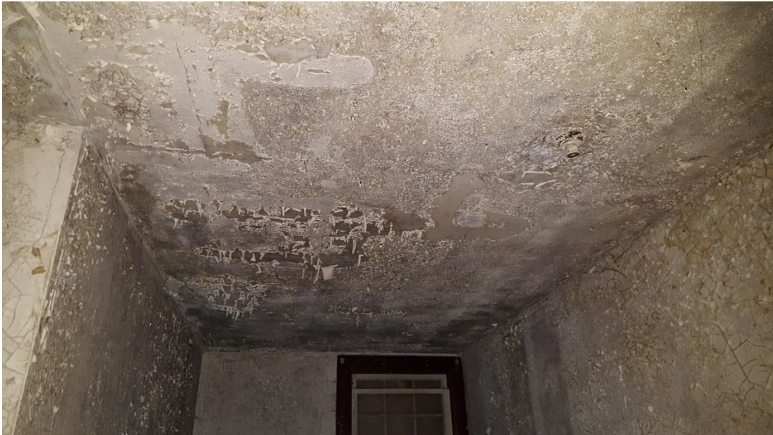
Figure 25: Extensive moisture infiltration in the ceiling of the second level at the staircase (2017).
